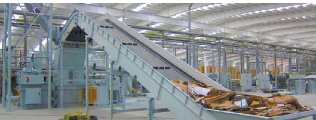
7 Scrap Handling Conveyors
